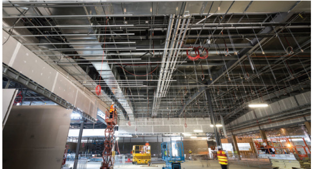
Using the Constructible Revit Model allows A.G. Coombs to make greater use of off-site pre-fabrication.
